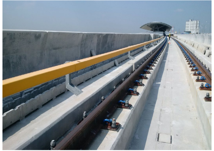
Third rail electrification
